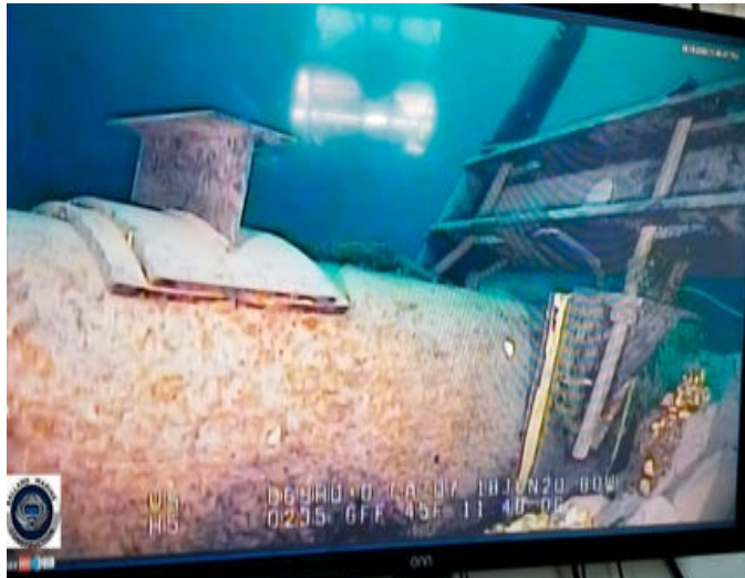
Damaged anchor support (right) holding East leg of Line 5 pipeline under the Straits of Mackinac
